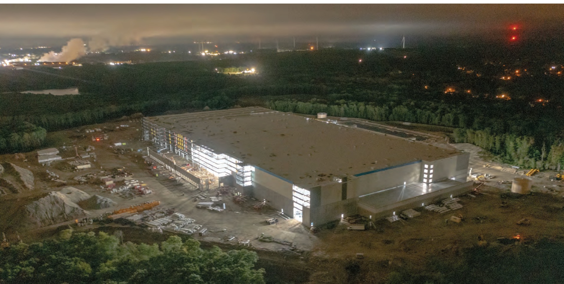
RIBBON CUTTING? According to Caitlin McLaughlin, Amazon Public Relations New England, the facility's completion date is scheduled for the "second half of 2023." The $290 million project is visible from points across the region, as crews work through the night.
